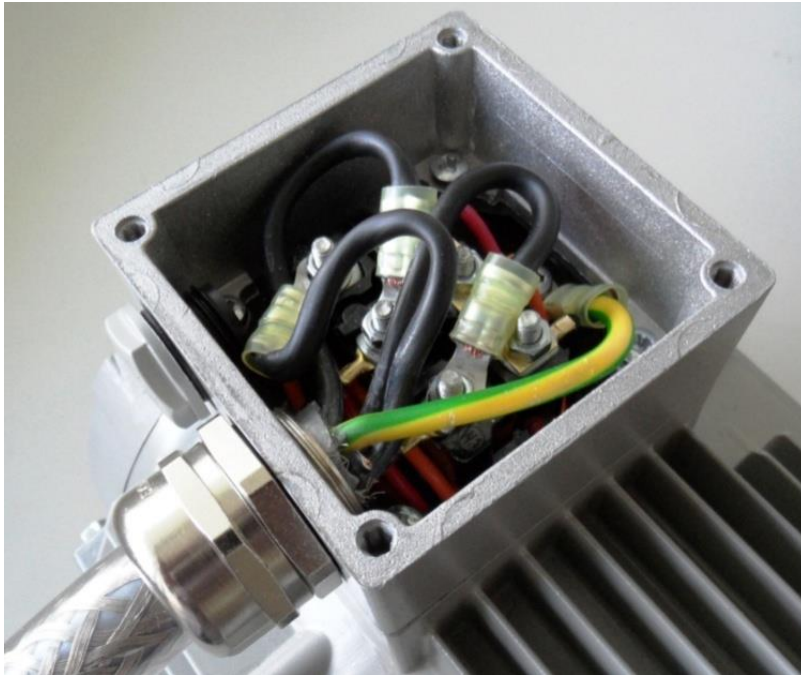
Fig. 20: Wiring on the motor connection box
