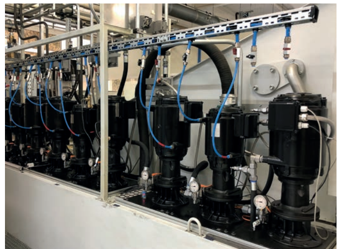
Noise reduction of the system by 8 dB(A) through water-cooled motors, despite the addition of three new pumps at the same time
